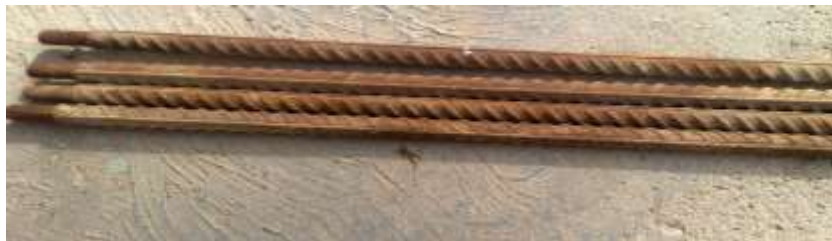
Plate( 1) the corrosion bars
